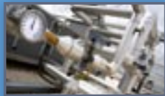
Boiler rooms and air conditioning
